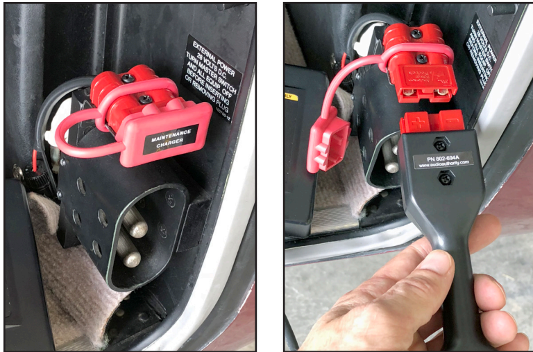
Figure 5. Finished installation example.
